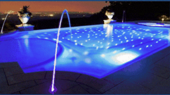
Fiber Optic Pool Lights
